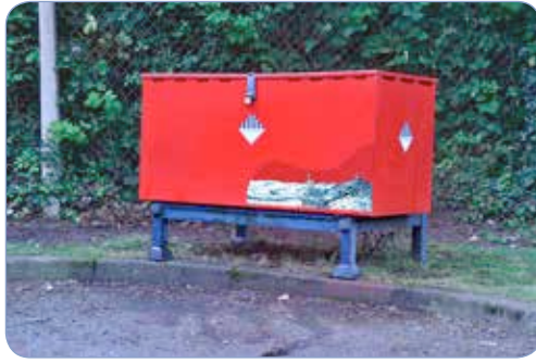
An example of a waste battery storage bin well away from buildings.
